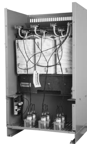
Guard II Transformer, (front panel removed)
